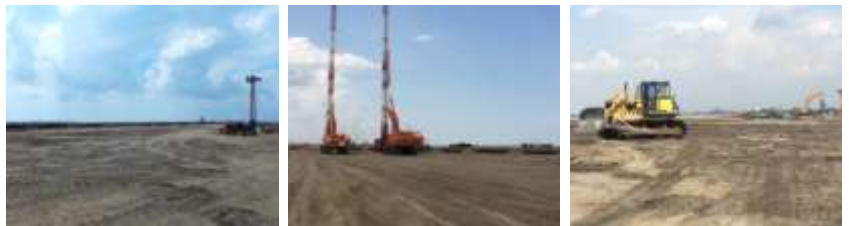
Sea reclamation is proceeding. Currently, the newly formed island for 1 st stage of port is around 40 ha.
